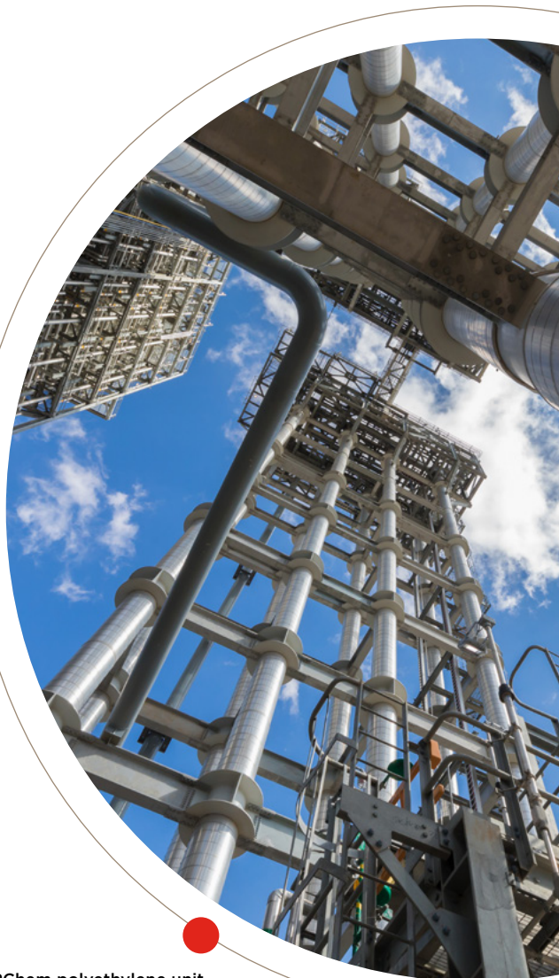
CPChem polyethylene unit OLD OCEAN, TX
