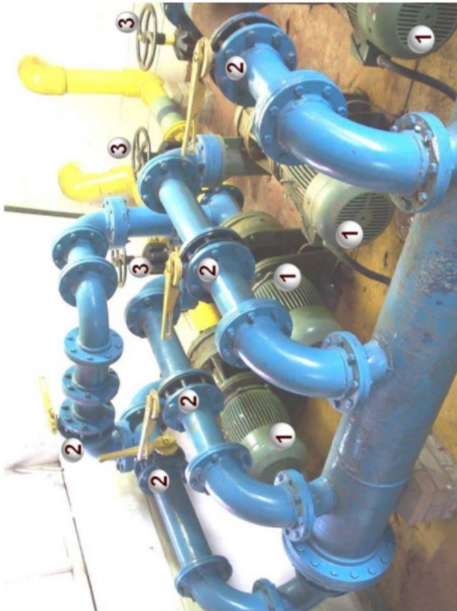
Exhibit 6.7 - Photograph 5: supply flow pumps
