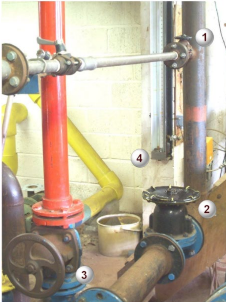
Exhibit 6.5 - Photograph 3: test control valves
