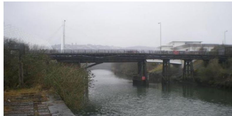
Morfa Bridge (also known as the Bascule Bridge), Normandy Road, Bonymaen - condition: Extreme Risk
