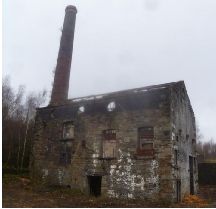
Vivian Engine House, Yorkshire Imperial Metal Works - condition: Extreme Risk
