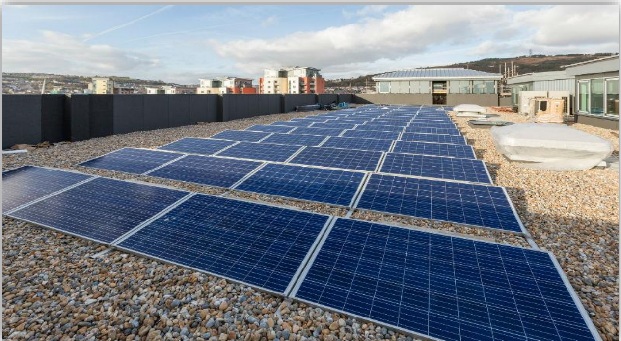
Figure 7: Solar PV currently implemented onto the IQ building in UWTSd's SA1 Campus ( Davies, 2017 ).
