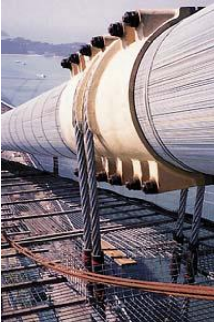
1.1m Diameter cable
