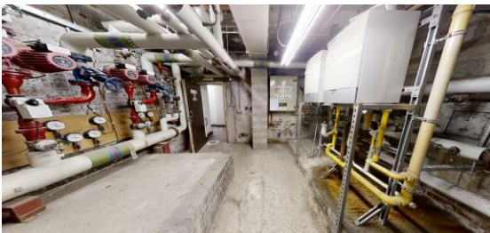
Image 10 A 3D scan of the boiler room of Y Cambria showing the upgrades and equipment (Theological College) (Aberystwyth University, 2023)
