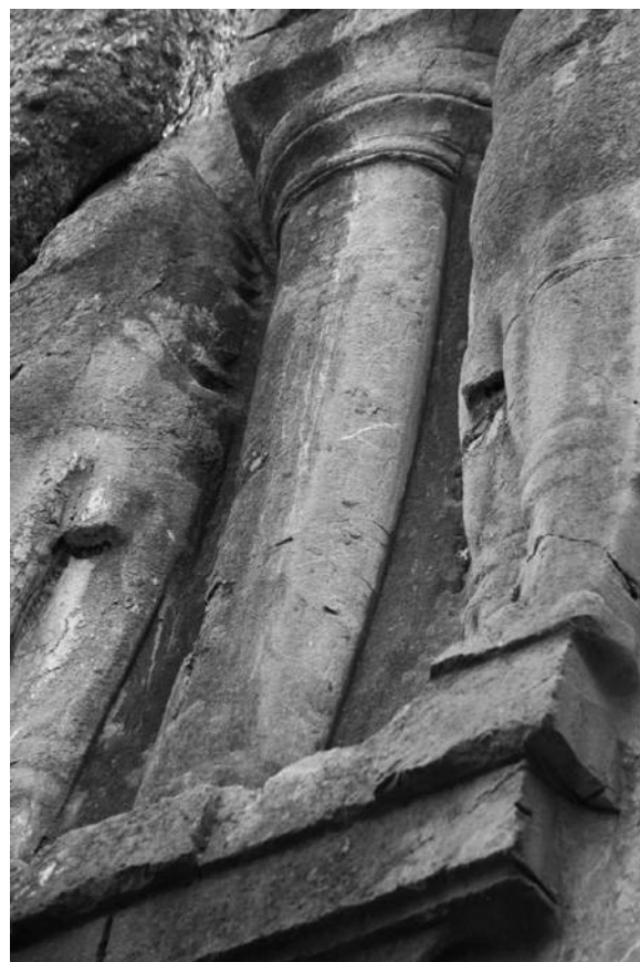
Fig. 10. Detail of the right side of column, cut by a pendulum saw.
