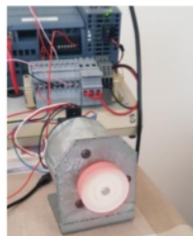
Figure 99 - PLC Motor Input
