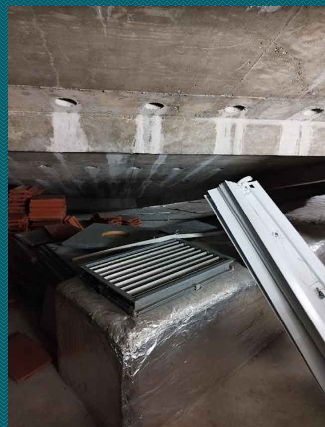
Air heating on one side, wet system on the other
