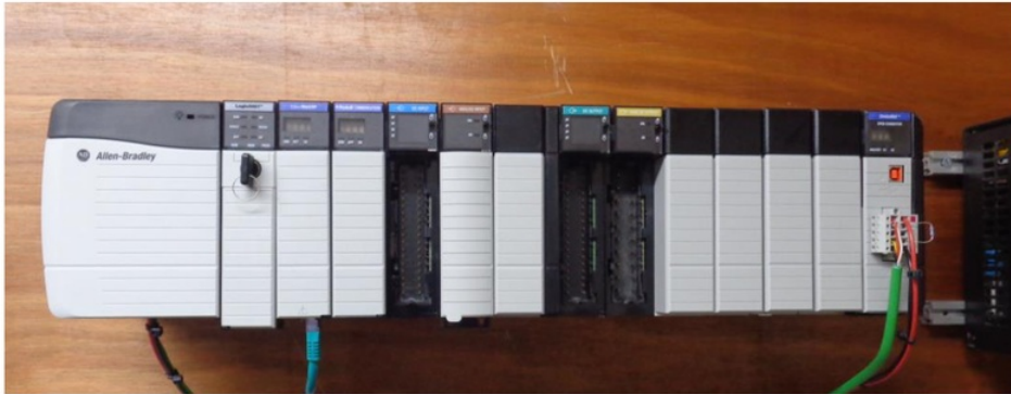
Figure 14: Allen Bradley ControlLogix PLC used for project
