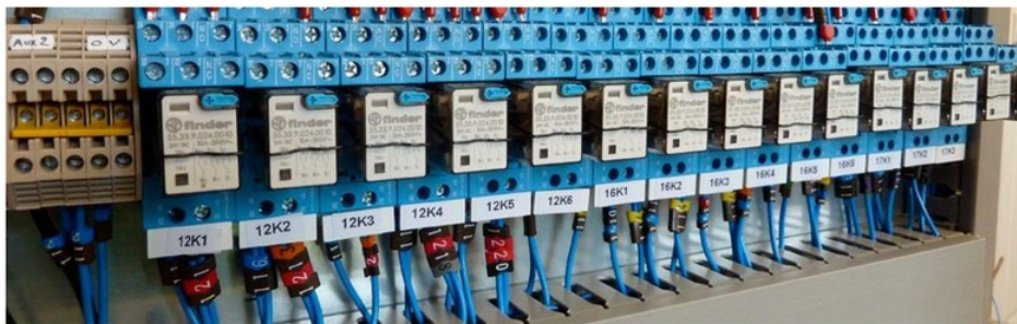
Figure 11: Example of a control panel consisting of relays (Small Panels, 2018).
