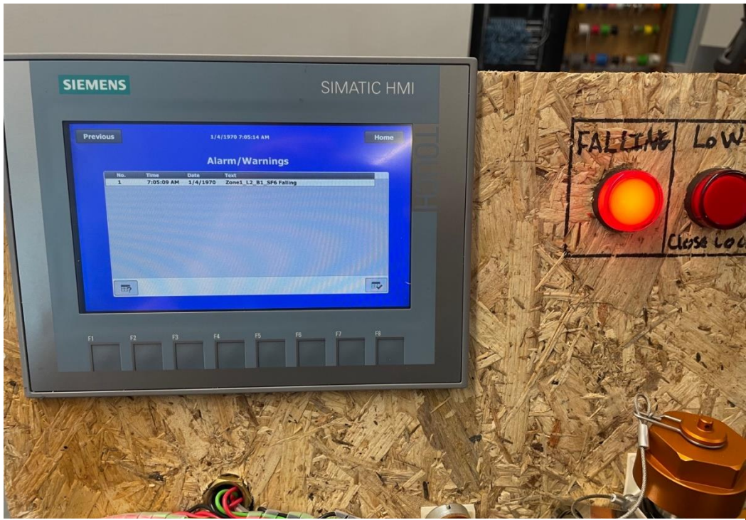
Figure 34: Alarm or warning screen with SF6 warning notification
