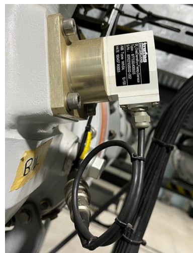
Figure 8: Existing Sensor installed on site
