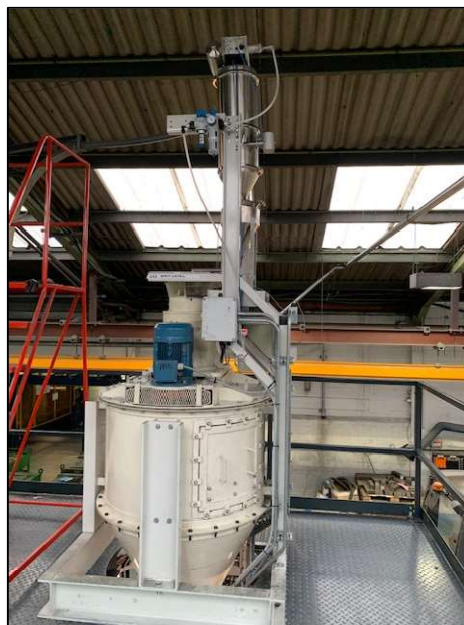
Figure 59 - Air Classifier Installed
