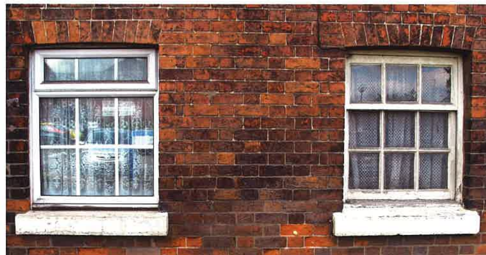
Permitted development rights Unsympathetic replacement window installed in an unlisted dwelling in a conservation area under 'permitted development rights'. This is an all-too-common sight in conservation areas where permitted development rights have not been curtailed by 'Article 4 direction'.
