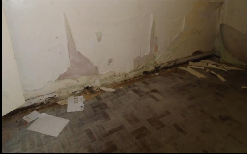
PAINT PEELING AS IF THE TIDE HAS COME IN, YET WE ARE 100 METRES ABOVE SEA LEVEL.
