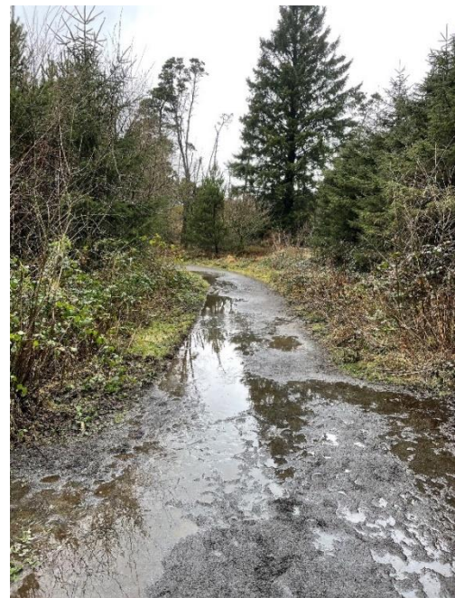
Figure 34 Example of surface water on path 2 (Egan, 2023)
