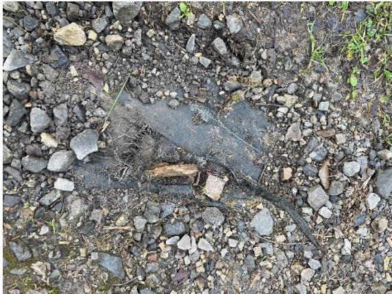
Figure 29 Example of damaged path in need of repair (Egan, 2023)
