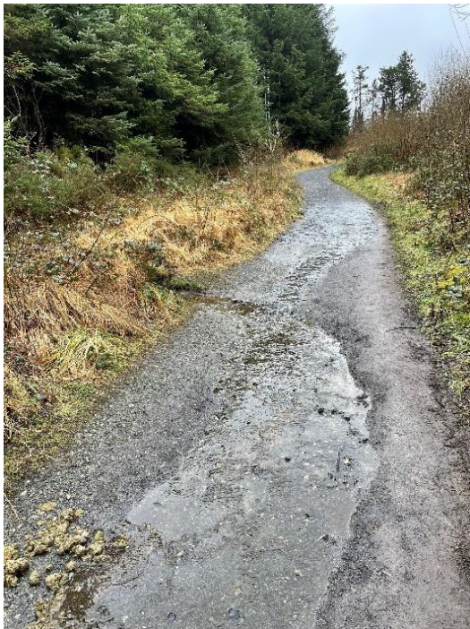
Figure 33 Example of damage on path caused by surface water 2 (Egan, 2023)
