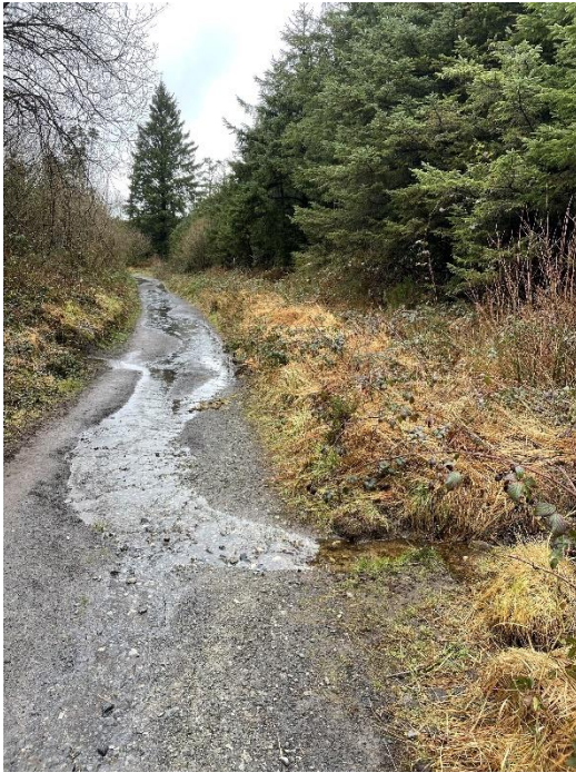
Figure 31 Example of surface water on path 1 (Egan, 2023)
