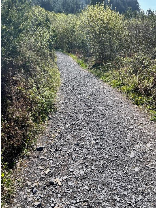
Figure 27 Example of path damage from water run off (Egan, 2023)
