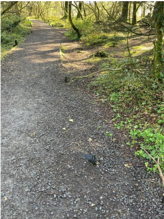
Figure 17 Example of drainage found on site (Egan, 2023)
