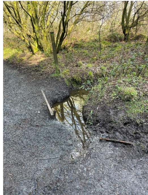
Figure 32 Example of damage on path caused by surface water 1 (Egan, 2023)
