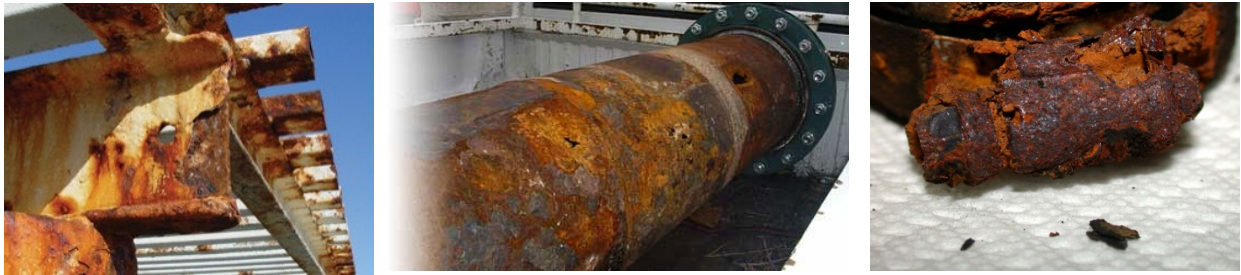
Figure 2: The corrosion of steel under various environmental conditions.
