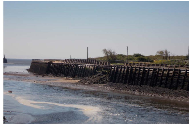
Damage to Swansea Inner West Pier retaining wall (ABPmer, 2018)
