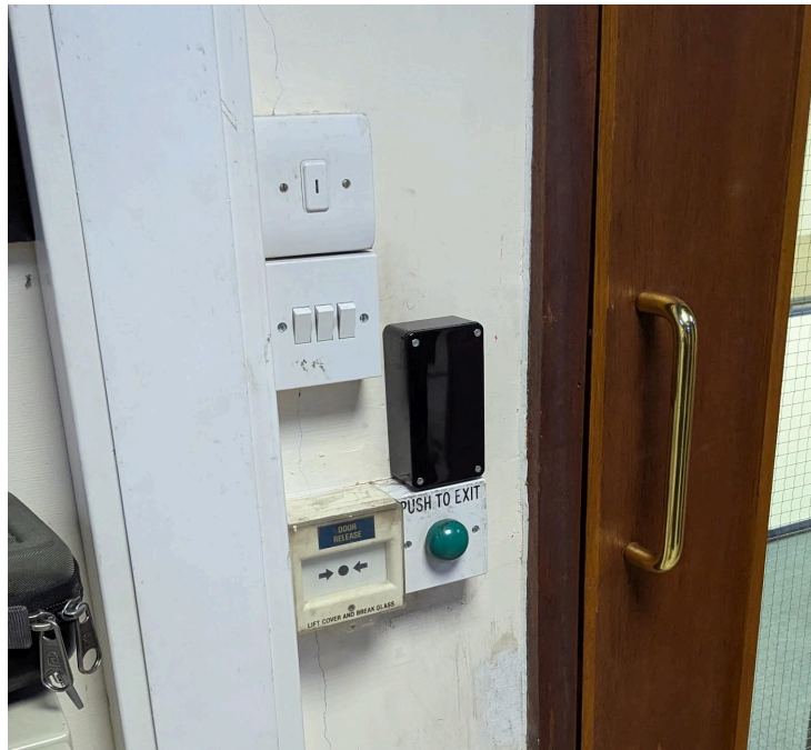
Figure 71 - Final Installation Back
