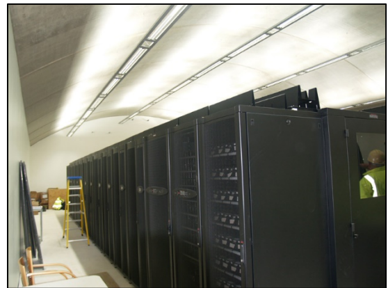
Figure 7: Server room at Renault F1 CFD facility.
