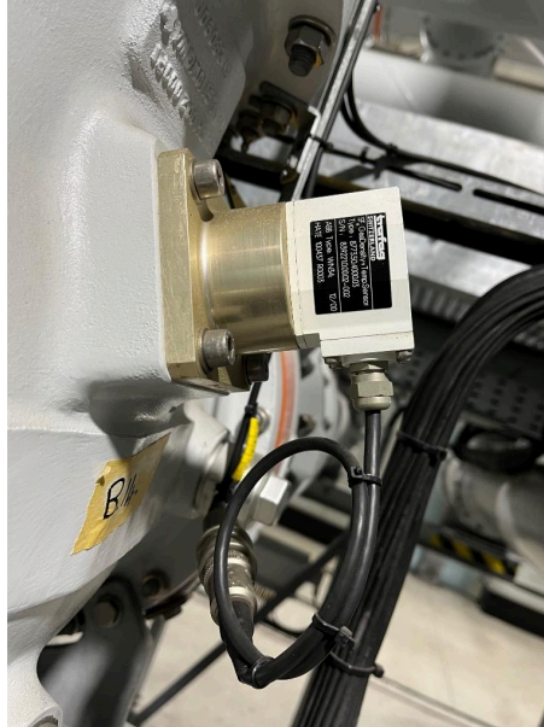
Figure 1 Existing Density Sensor
