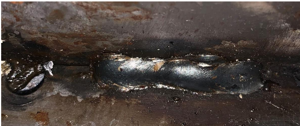
Figure 5 – Example of the lack of fusion on a weld called 'Cold lap'.
