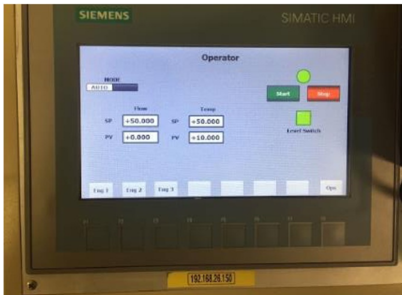
Figure 29: Operators HMI screen
