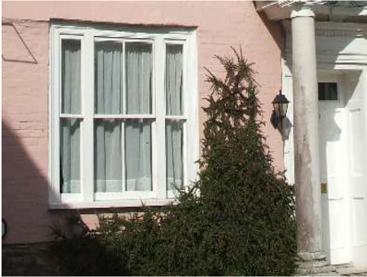
Figure 1. Traditional sash windows, fitted close to the face of a wall. Details that were challenged by their performance in use and fire safety issues.
