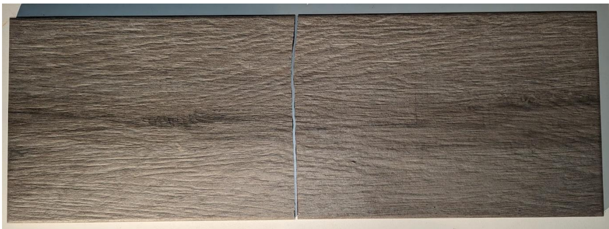
Figure 39 Ceramic floor tile after failure
