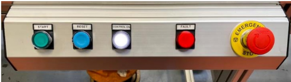
Figure 52 – Operators Control Station
