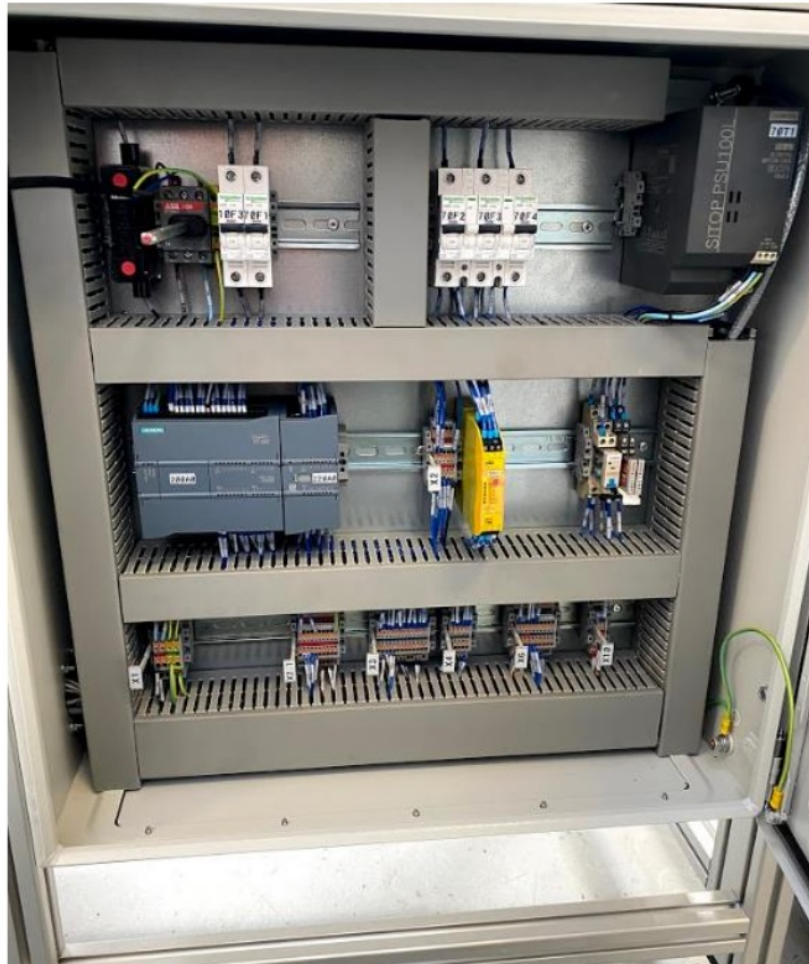
Figure 49 – Control Panel inserted into Cabinet
