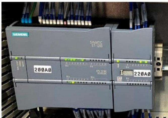
Figure 76 – PLC I/O Illuminated during testing
