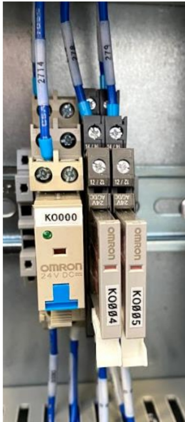
Figure 47 – Electromechanical Relays Wired
