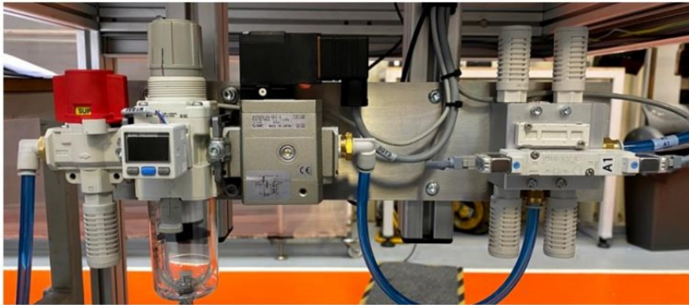
Figure 51 – Air Service Unit
