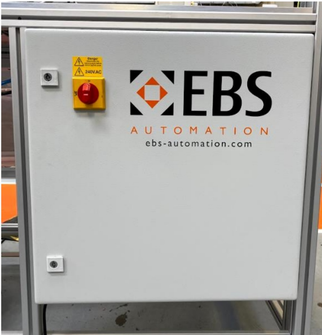
Figure 58 – Control Panel with Isolator and Warning labels
