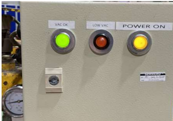
Figure 31 – Vacuum Ok LED ON
