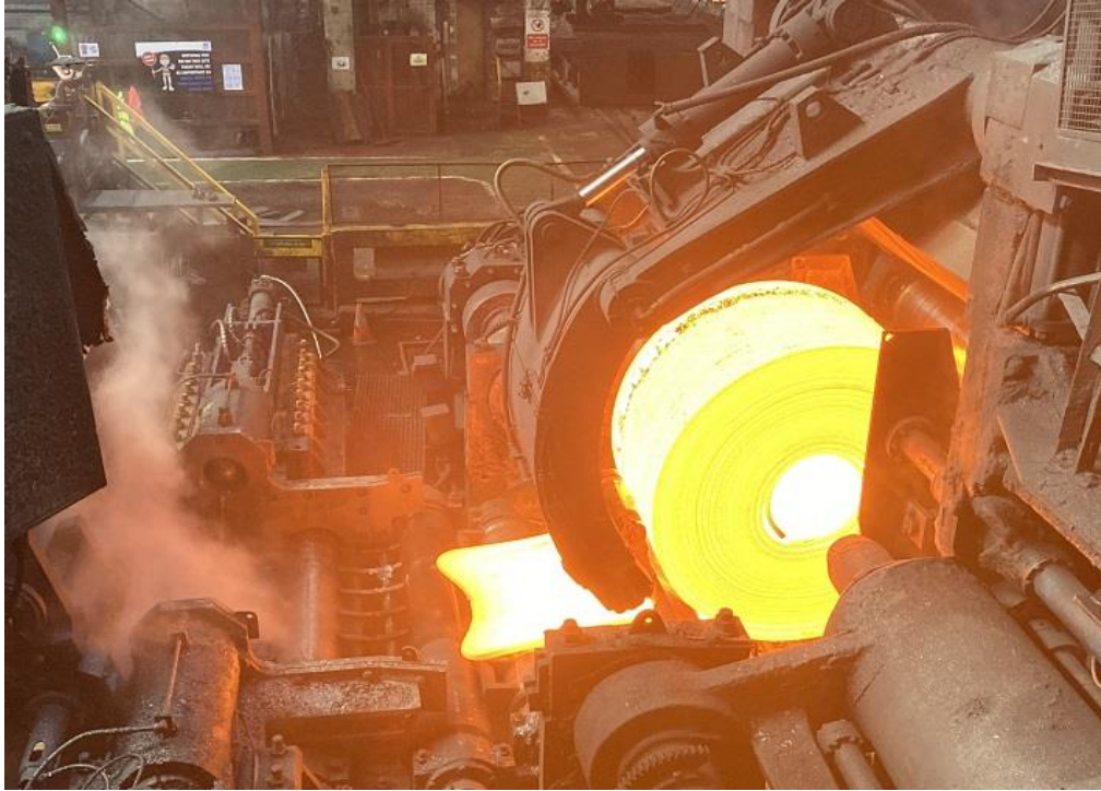
Figure 21 - Coil Box feeding a transfer bar into the finishing mill stands
