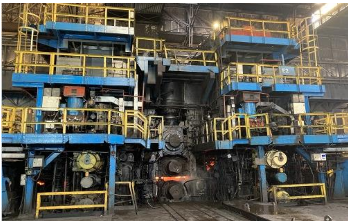
Figure 18 - Reversing Roughing Mill at HRP
