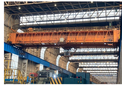
Figure 5. AA115 cold mill crane
