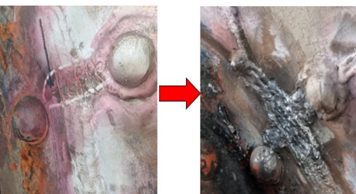
Figure1. Crack in AA115s structure weld repaired
