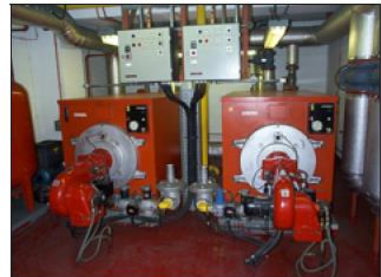
Example of forced-draught gas boilers.
