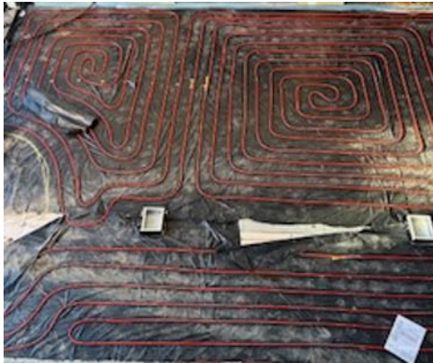
Figure 4 Showing underfloor heating installation
