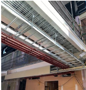
Figure 10 Showing Metal Carry Trays for M&E
