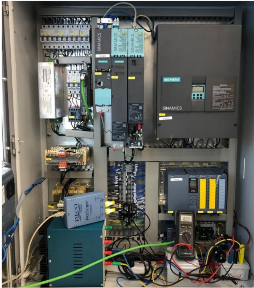
Figure 6: Drive cabinet contents
