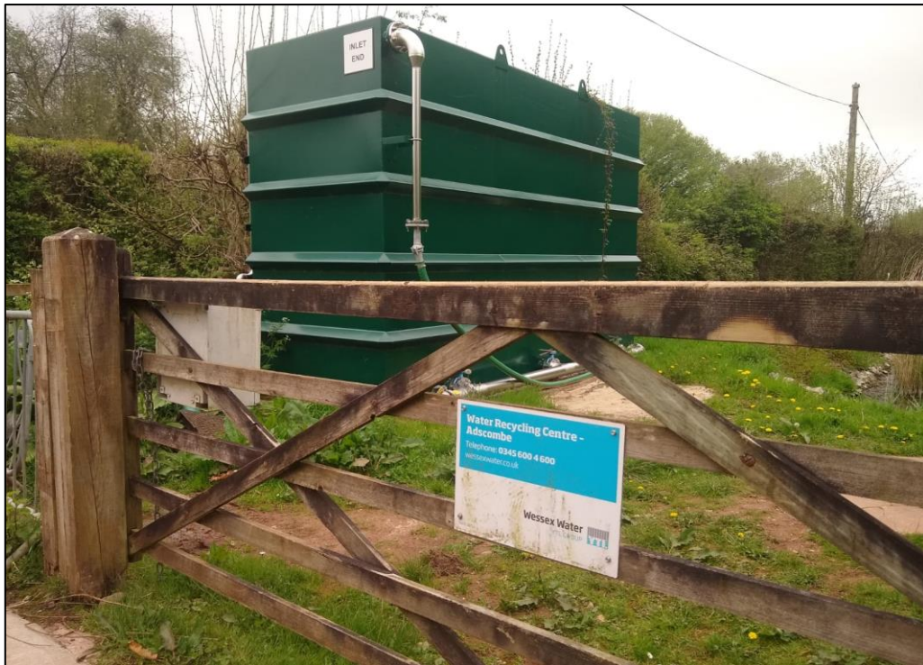
Figure 5. Water Recycling Centre below the chapel field, Adscombe, May 2023. Photo: Dan Broadbent.
