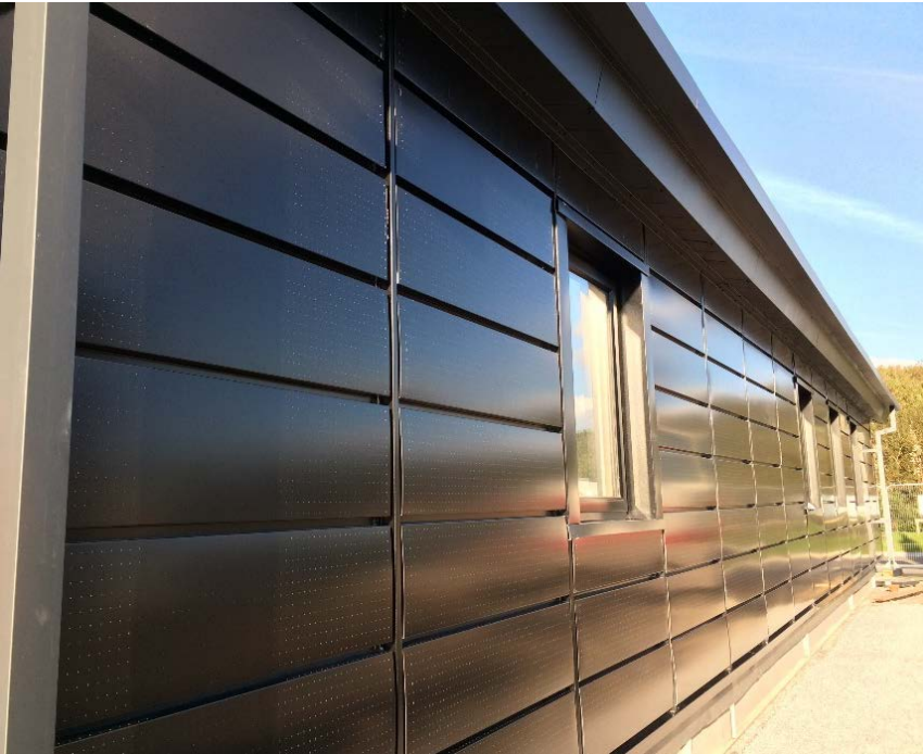
Two transpired solar air collectors, Tata Colorcoat Renew SC ® :
