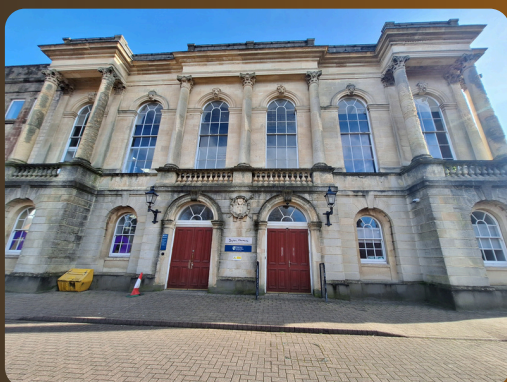
Figure 1 – Building Exterior / Façade The existing external façade shows signs of ageing, which may contribute to thermal inefficiency and ongoing maintenance requirements.(King, 2026)
