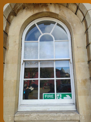
Figure 2 – Windows Condition Some elements of the building envelope where heat loss and material deterioration may occur. (King, 2026)
