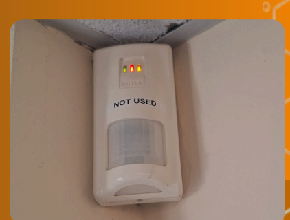
Figure 6 – Motion Sensor A example of installed but unused smart technology, demonstrating the gap between system installation and effective utilisation. (King, 2026)
