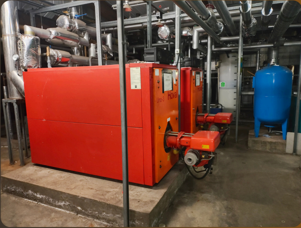
Figure 10 – Boiler Plant Room the building relies on traditional heating systems, which may be inefficient compared to modern alternatives. (King, 2026)
