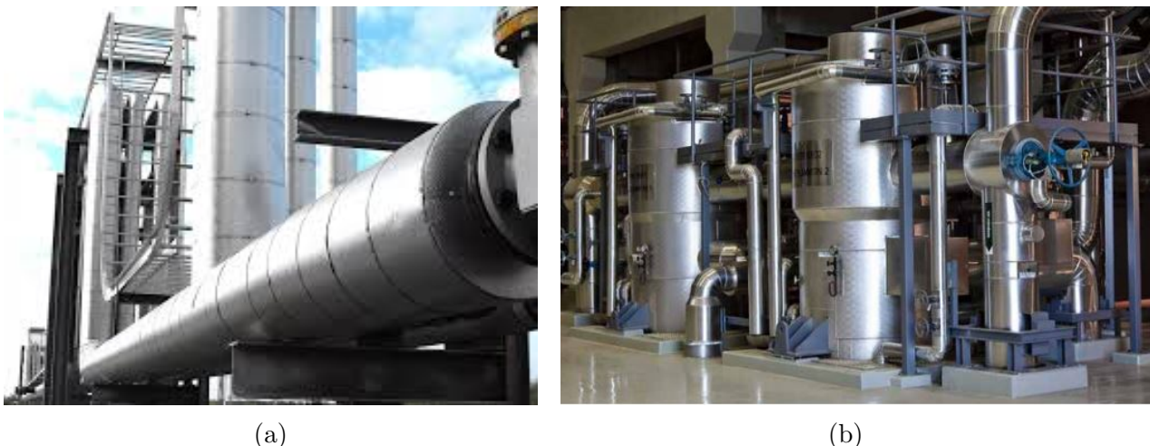
Figure 2.2: a) Insulated pipework and b) Insulated vessels
