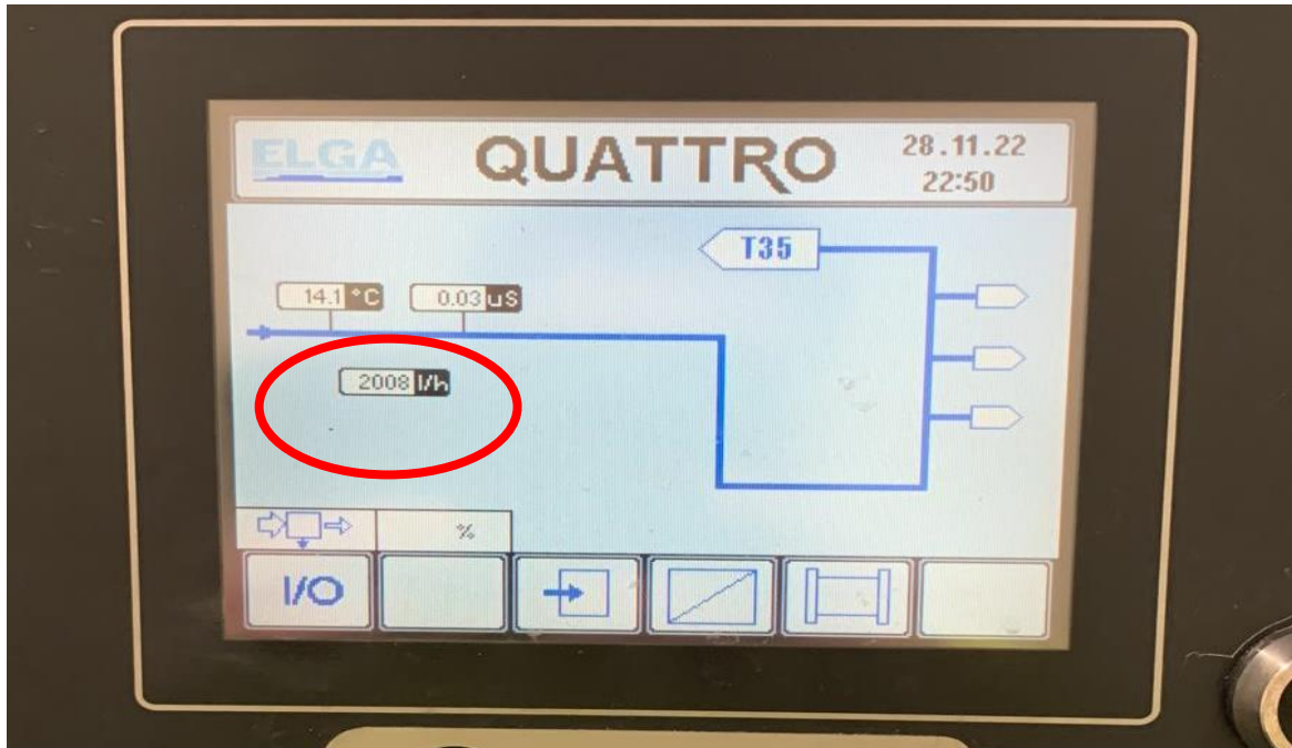
Figure 57 Quattro control panel screen 3 highlighted 2,008l/h output and a recirculation line back to the storage tank. Monitoring temperature and conductivity.
