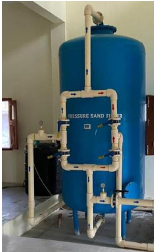
Figure 24 Pre-treatment sand filter unit after re-charge
