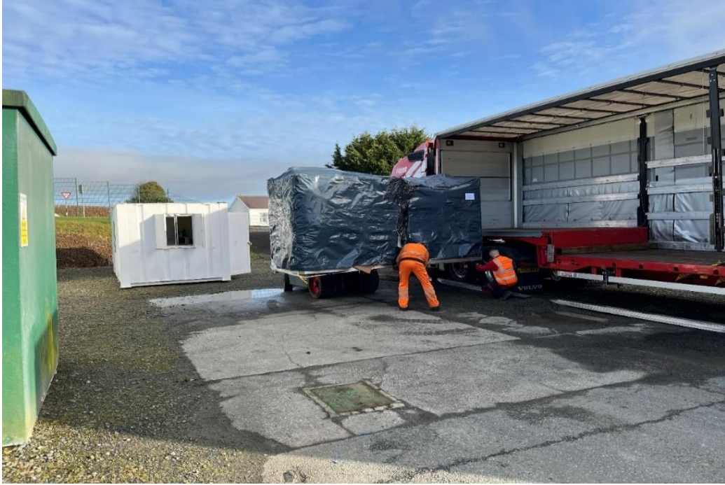
Figure 37 Delivery of the Orion 4000 plant
