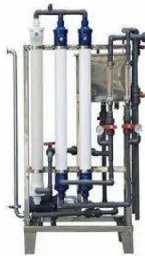
Figure 11 Ultrafiltration unit in operation
