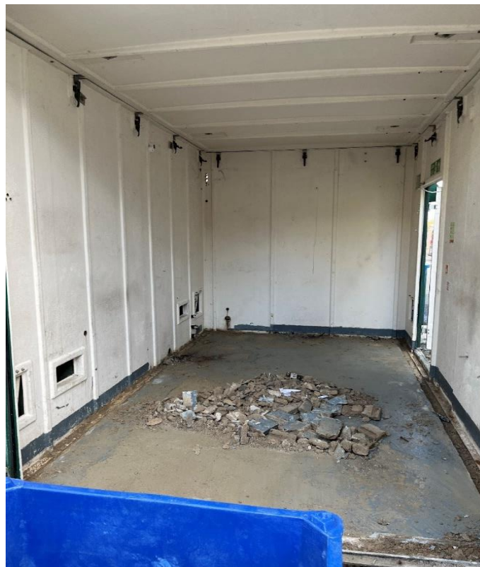
Figure 29 The glass reinforced plastic enclosure empty, and utilities removed
