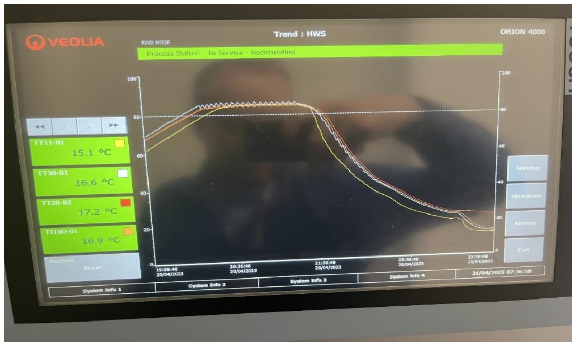
Figure 59 Orion control panel trending temperature data
