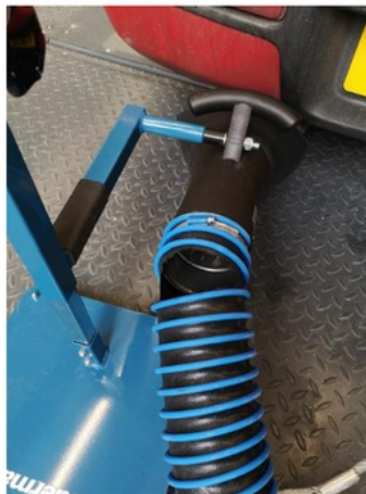
Figure 17 Photograph showing failed exhaust extraction hose
