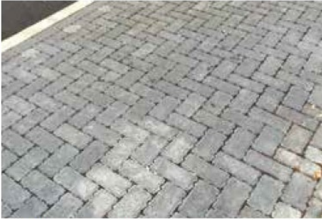
a Block permeable paving
