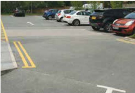
c Porous concrete
