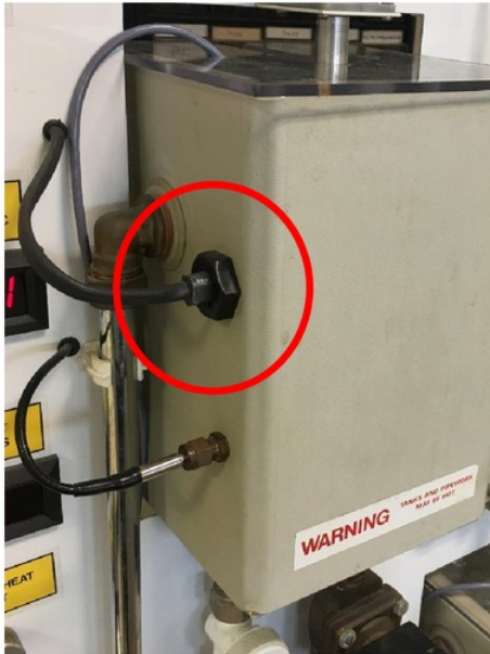
Figure 18- Float Switch Outside Tank
