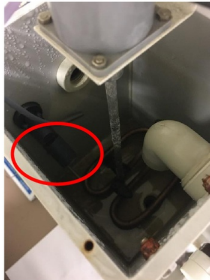
Figure 19- Float Switch inside Tank
