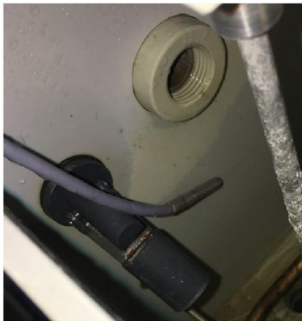
Figure 5- Process Tank RTD
