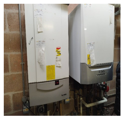
Twin Boiler set up (Modular)
