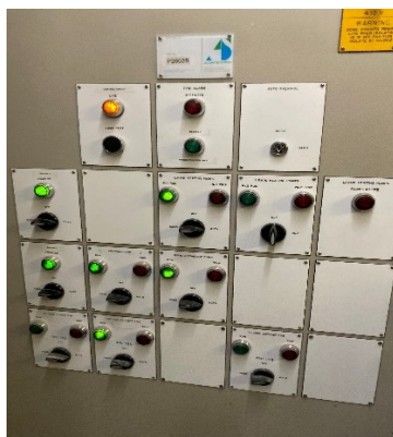
Switching Control Panel
