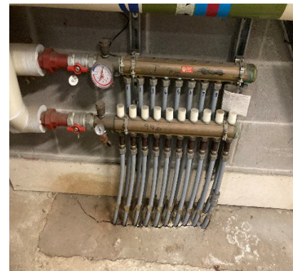
Under Floor Htg. Manifold
