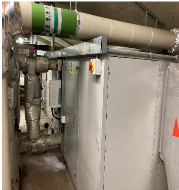
Air Handling Unit
