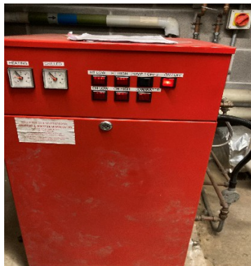
Htg. & Chilled Pump Set
