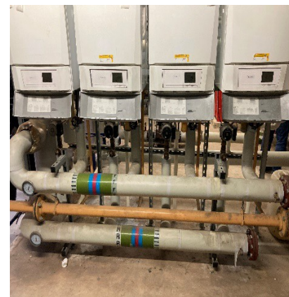
Four Boiler set up (Modular)
