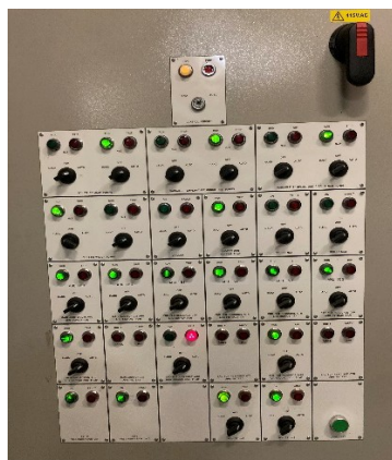
Switching Control Panel
