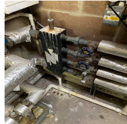
Low Loss header supply
