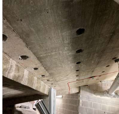
Vents to Lecture Theatre
