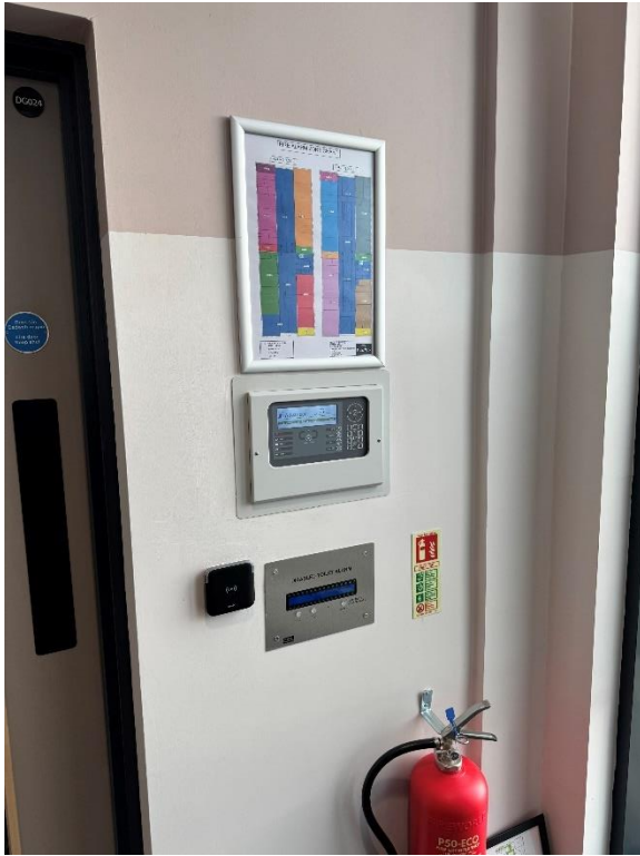
Figure 7 Fire and BMS
