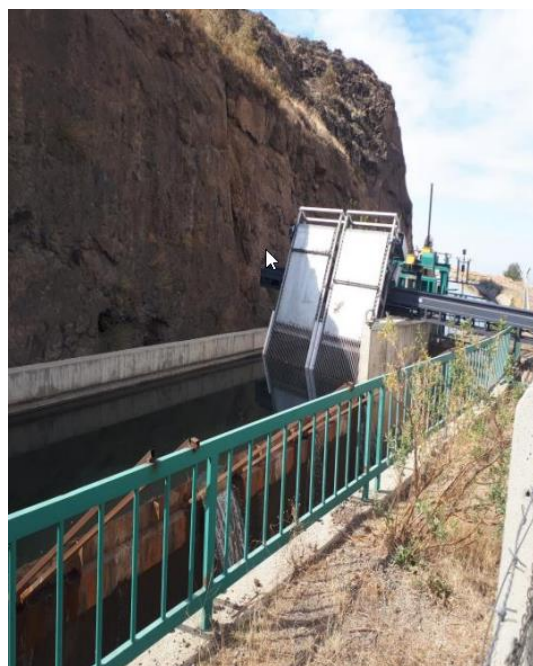
Figure 2: Mechanical bar screen used in field.
