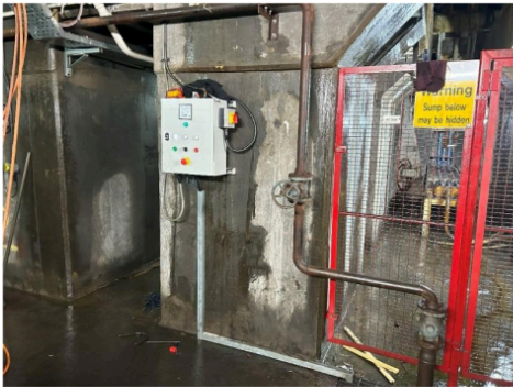
Figure 21 - Sump Pump Cable Unistrut
