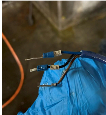
Figure 20 - Sump Pump Cable
