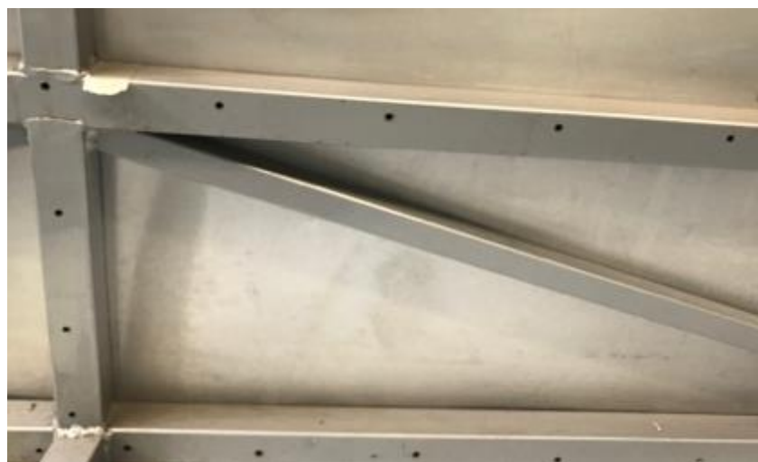
Figure 11 Chassis bars showing drilled holes.
