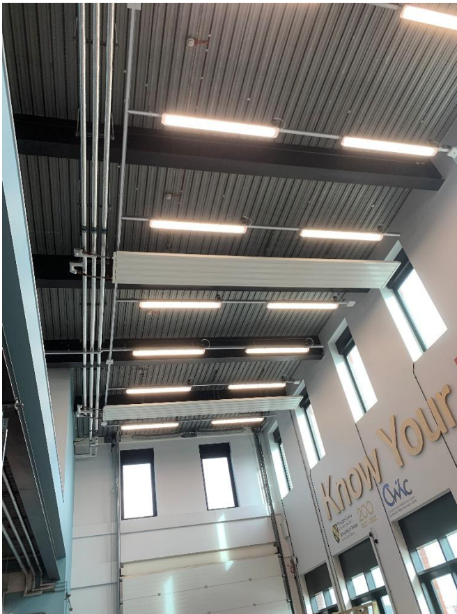
Figure 2 Image of the CWIC workshop heating system (Burgess, 2026)
