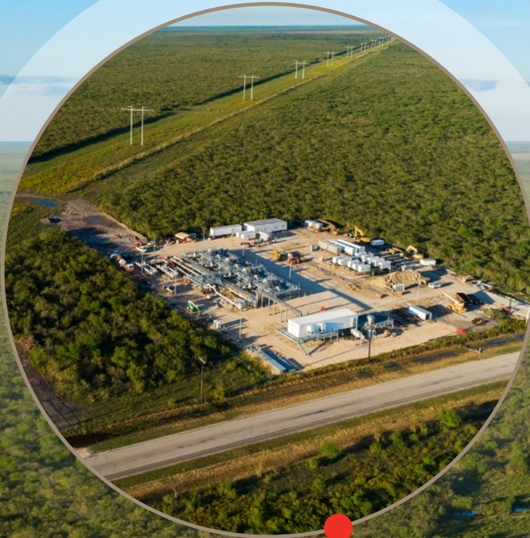
C2G Pipeline REFUGIO, TX
