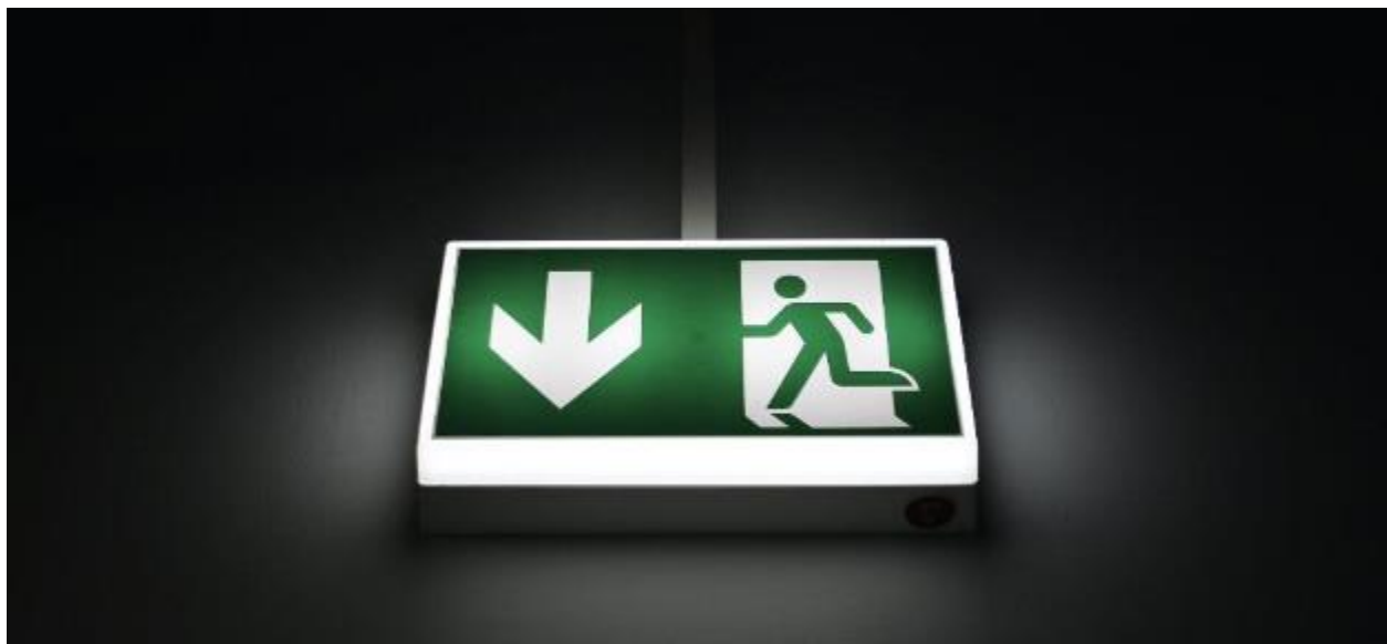
Fig 2 (FMC Fire, 2022, Fire Exit Sign)
